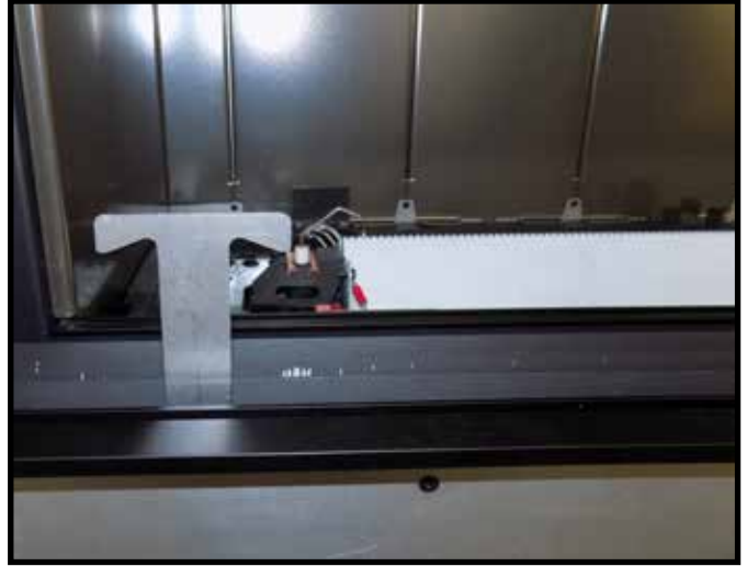
Figure 31: Gas valve shut off.
