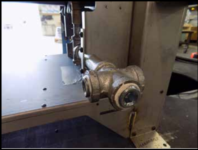
Figure 30: Gas connection point.
