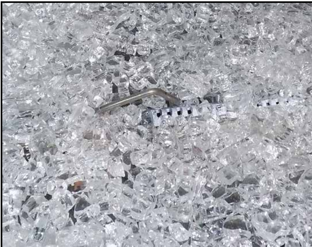
Figure 34: Exposed holes beneath the igniter.
