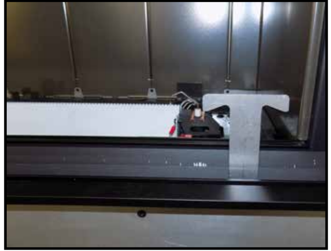
Figure 31: Gas valve shut off.
