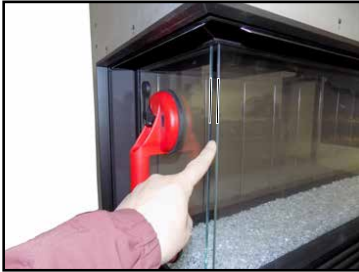
Figure 46: Gap present before sliding left side glass panel to the front.
