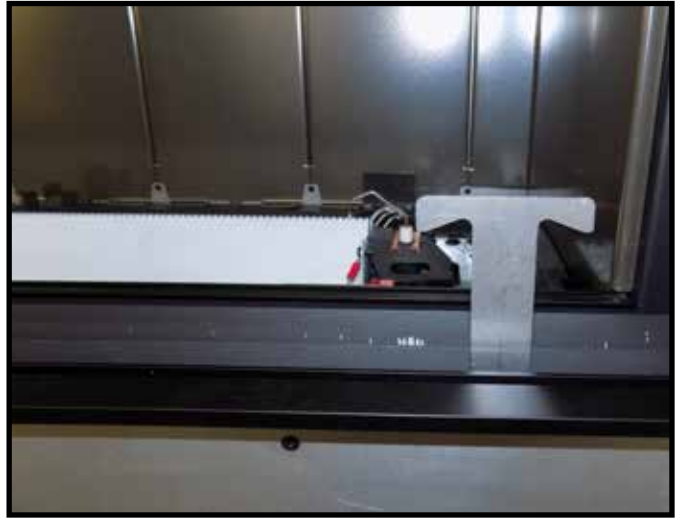
Figure 65: Gas valve shut off.
