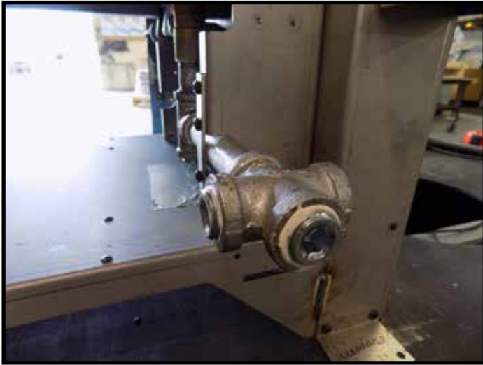
Figure 64: Gas connection point.
